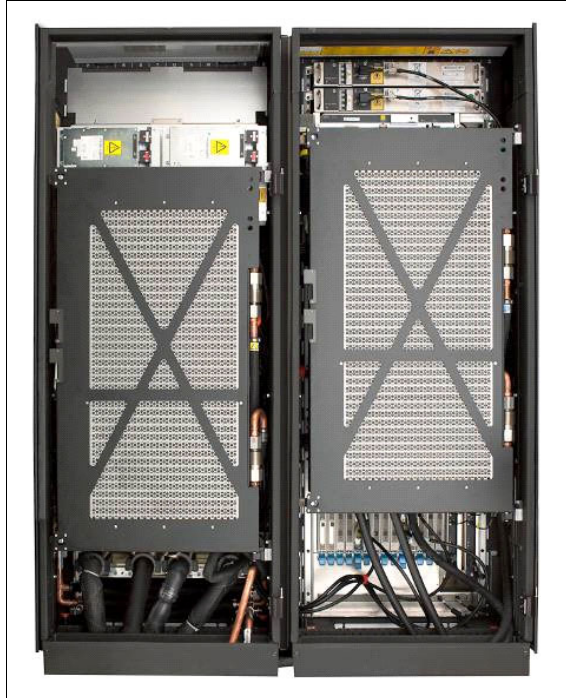
Figure 2-32 Water-cooled model: Rear view
